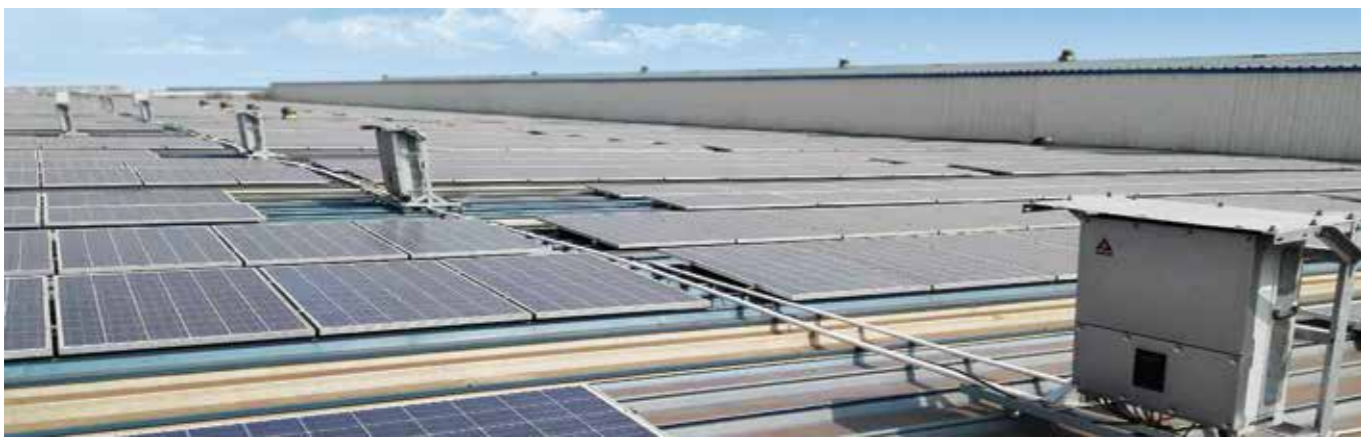
ASP-30KTLC, ASP-20KTLC for 5MW distributed solar power station at MCC Baosteel
