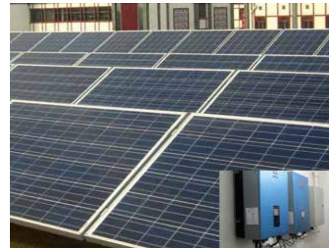
ASP-10KTLC for 20KW distributed solar power station at Weishan Jail
