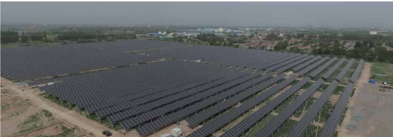
ANBF-1000KTL for 20MW solar power station at Jilin
