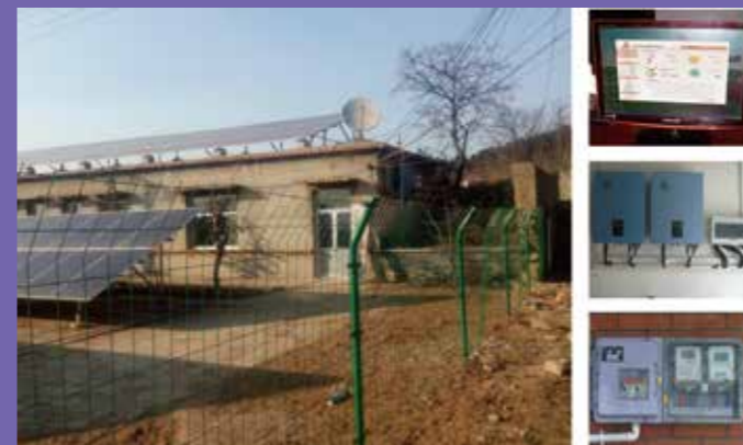
Poverty Relief PV Power Projects at Pingyin County These projects are located at 14 villages. Total installation is 360kw, about 30-50kw at each village. All generated power is fed into the grid. Stable income every year is RMB39,000-65,000
