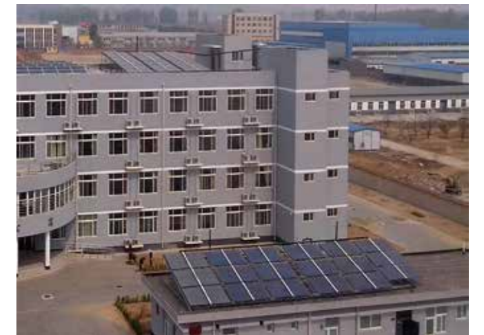
ASP-50K for 1.5MW Gold Sun Campus Roof Top solar power station at Beijing
