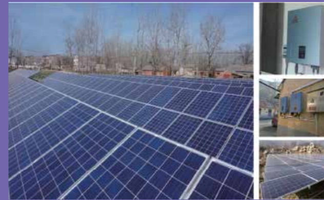
Poverty Relief PV Power Project at Laiwu Total installation is 300KW at 5 villages. All power generation is fed into the grid. People there have stable income every year.
