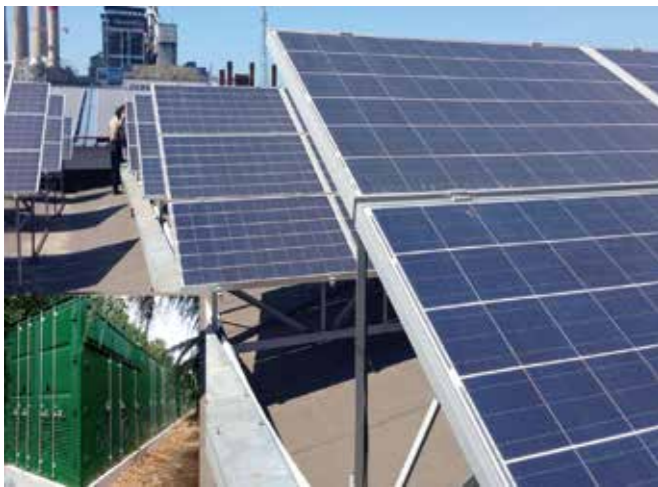
ASP-500K, ASP-630K for 7.158MW solar power station at Linuo Group, Shandong
