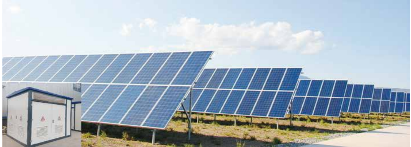
ASP-500KTL for 40MW solar power station at Weishan Xuri
