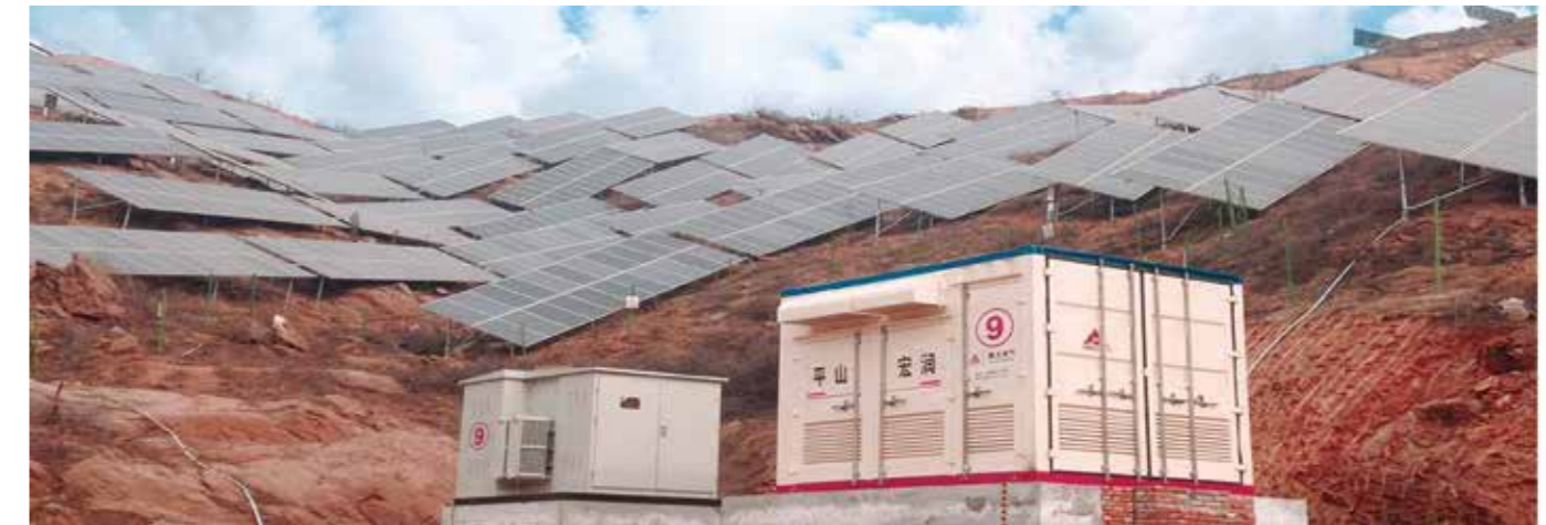
ASP-500KTL for 50MW solar power station at Pingshan, Hebei
