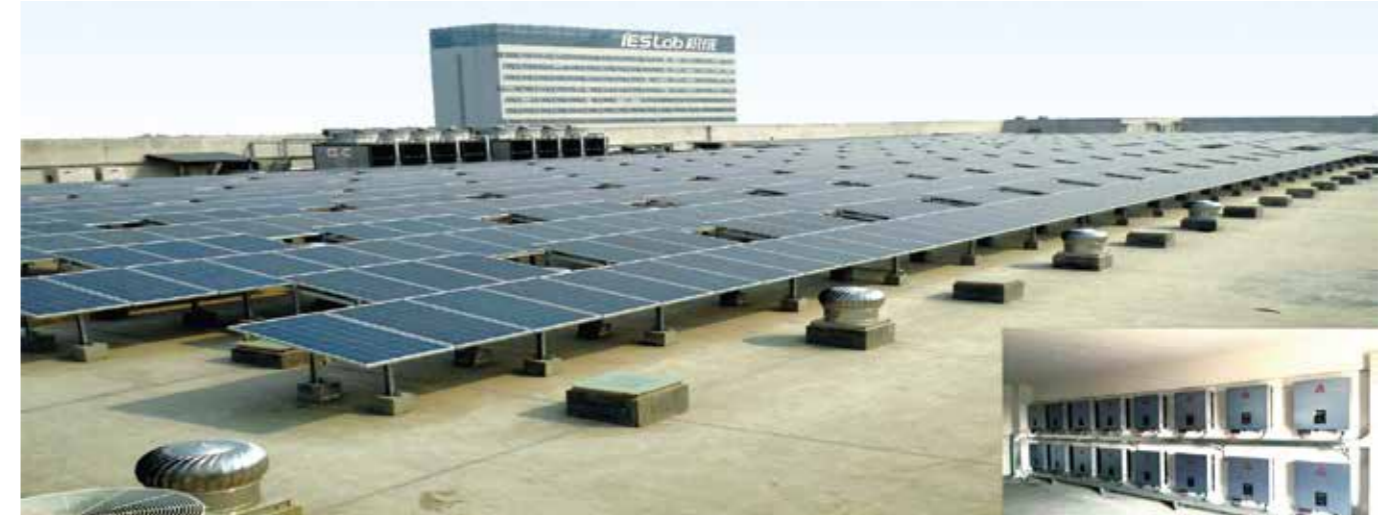
ASP-20KTLC for 320KW solar power station at Jicheng Electrical Park
