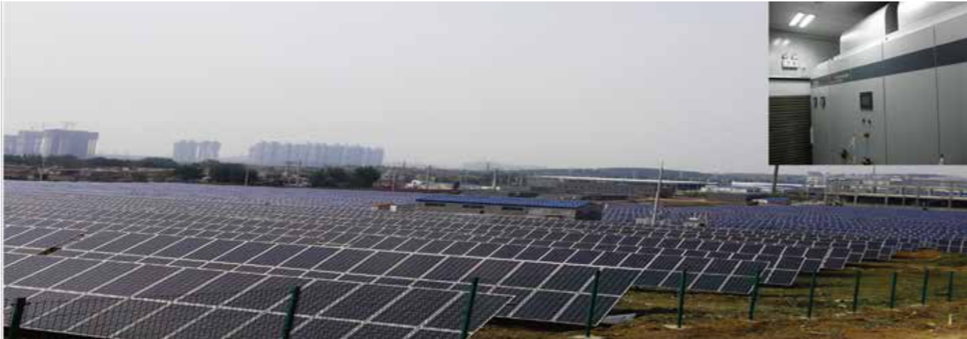
ASP-500KTL for 10MW solar power station at Shanghai Power, Fengxian
