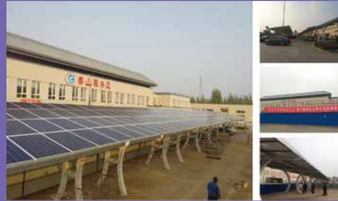
65MW Distributed PV projects at High-speed Service Areas, Shandong This project at Taishan high-speed service area is the first one for demo, total installation about 260kw.
