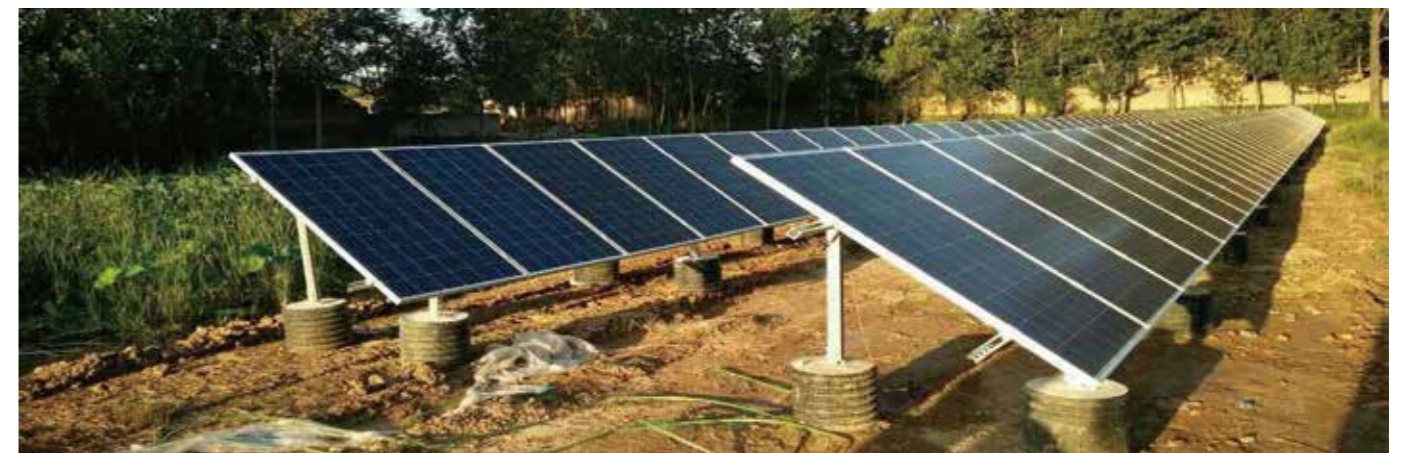
ASP-30KTLC, ASP-20KTLC, ASP-10KTLC for 8.5MW poverty relief PV power projects at Heze
