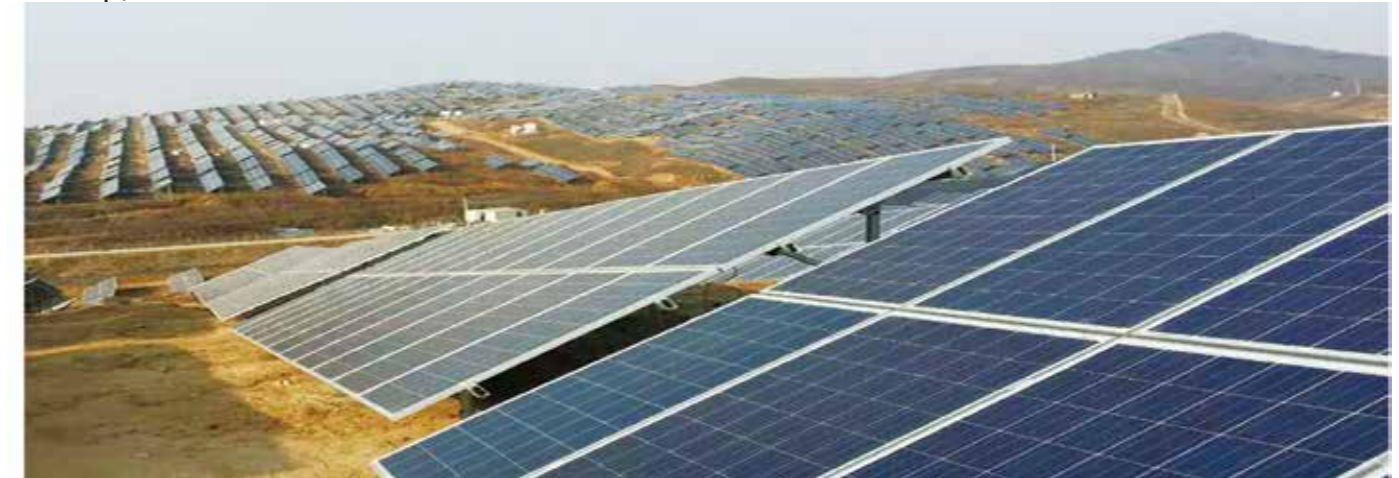
ASP-500KTL for 30MW solar power station at Taohuayu, Laiwu
